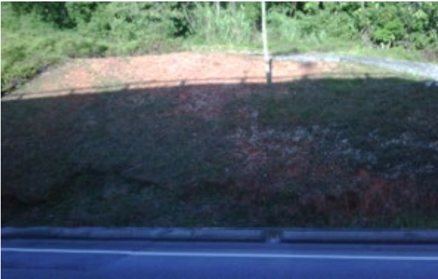
Figure 10: Eroding slope along a highway
