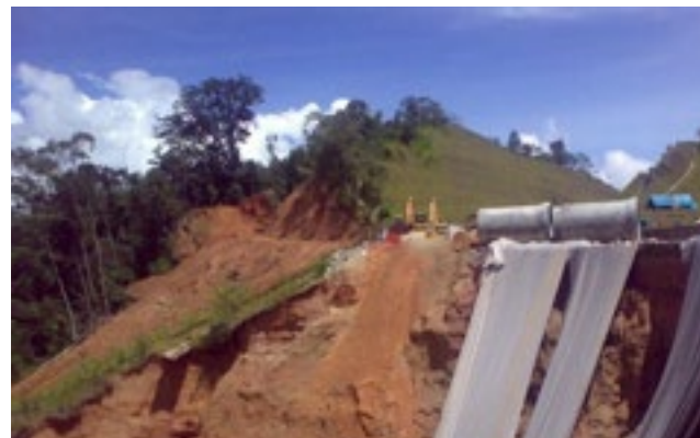
Figure 4: Slope failure, Lojing Highlands, Kelantan
