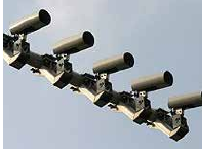
Figure 5.35 ANPR cameras mounted on a vertical pole
