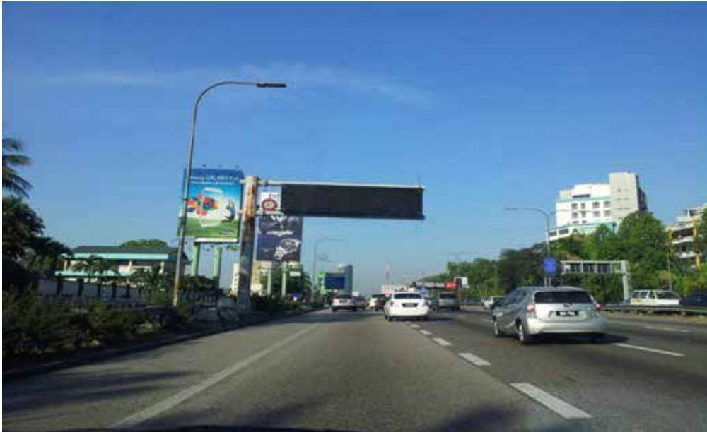
Figure 5.9 Dysfunctional ITIS Variable Message Sign Panel on Federal Highway in 2014
