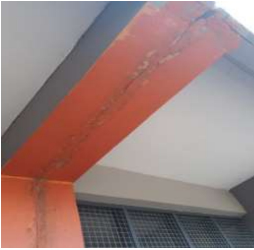
Figure 8: The damaged can be seen clearly and it isn't properly repaired
