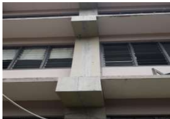
Figure 7: Damaged building in SK. Kundasang due to the recent earthquake
