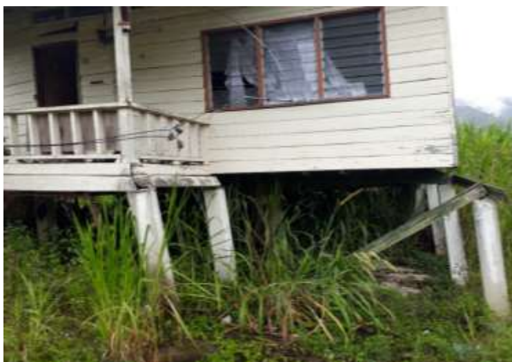
Figure 12: Extremely damaged house caused by the seismic activities in the area
