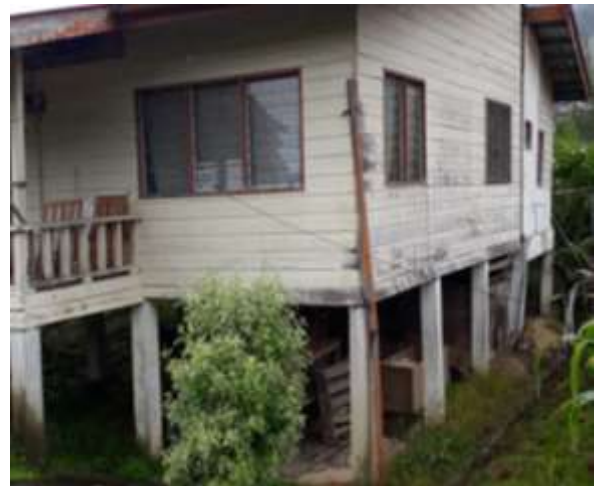
Figure 11: Damaged house in Kg. Mesilau due the seismic activities in the area
