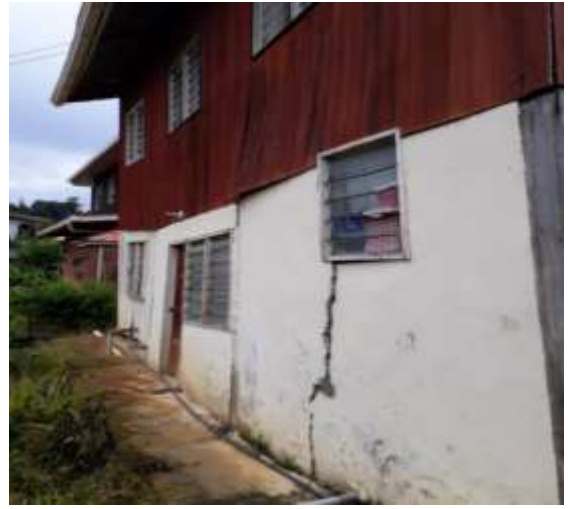
Figure 10: A house located in Kg. Lobou-Lobou Kundsang destroyed by the 2015 earthquake
