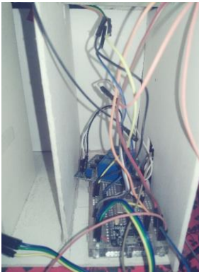
Figure 8. Controller and Relay setup
