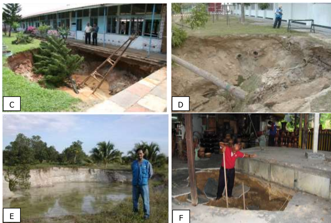
Figure 2. Sinkholes cases in the vicinity of Kinta Valley, Picture C - SMK Kopisan, Gopeng; Picture D - Institut Latihan Tentera Udara, Jln. Lapangan Terbang, Ipoh; Picture E - Kg. Kuboi, Gopeng (happened on 26/12/2004 after Aceh Earthquake); Picture F - Jalan Lahat, Ipoh.
